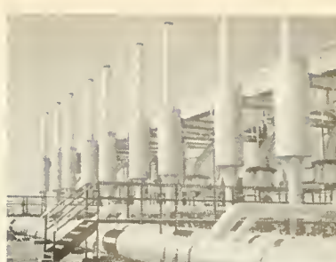
Natural gas booster station equipped with THE MAXIM SILENCER COMPANY'S devices.
